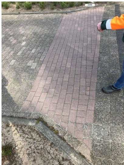
Figure 12. A piece of new street work. This road was so bad a few years ago that they laid it again. The broken bricks have been thrown away and for this last piece they were short of stones which they later supplemented with new ones.
