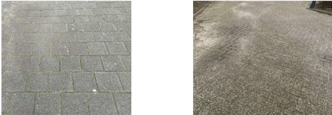
Figure 8 and 9 Pavement in the area of Griffiersveld (see also Appendix I).
