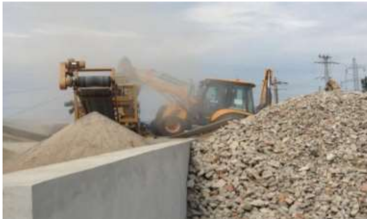
Figure 13. A concrete crusher at a depot in Romania. Here a dumper is being used to transport the bricks into the crusher. (Deloitte, 2016)
